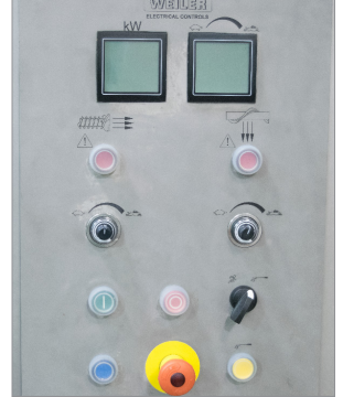
VARIABLE SPEED CONTROLS
